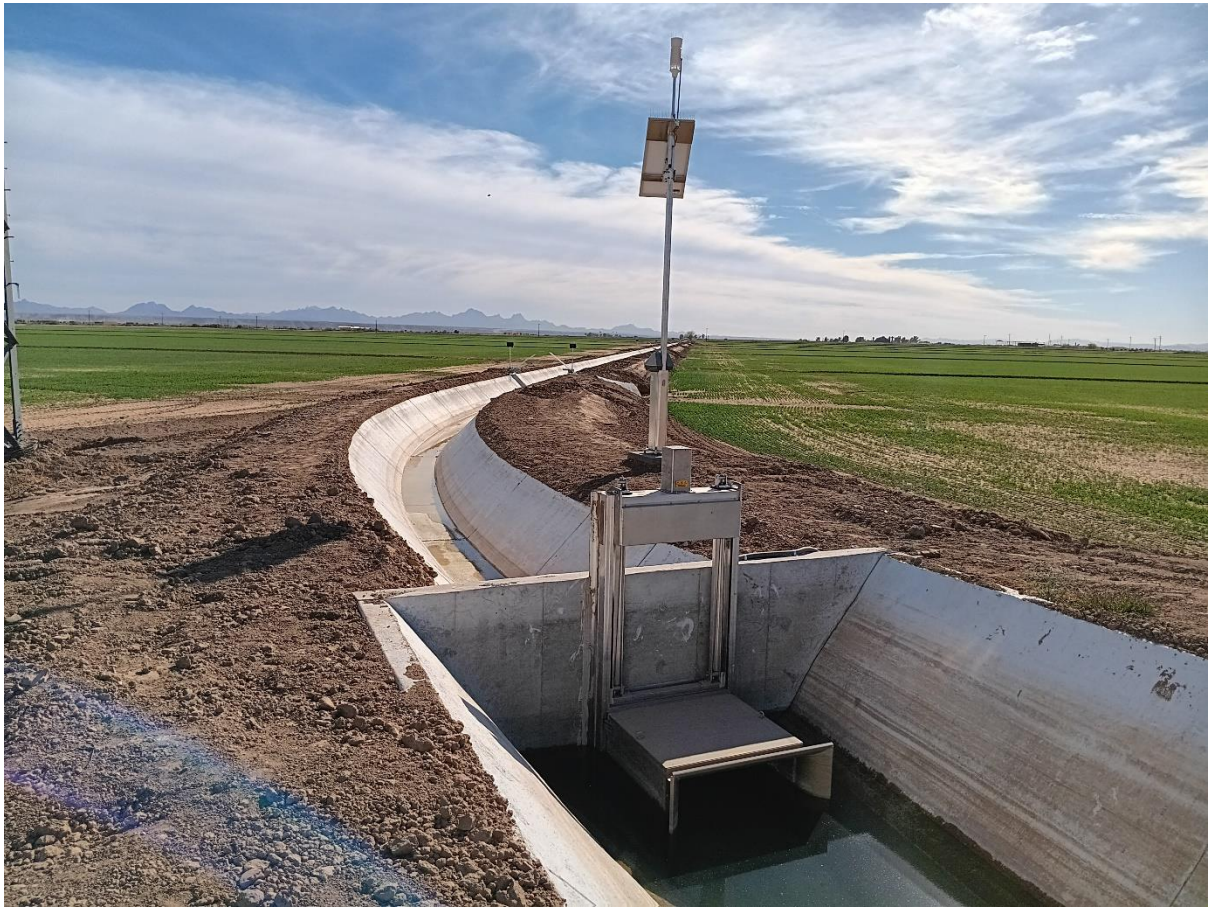
Figure 13 AgPod Smart Meter connected to a Farm Turnout flowmeter (SlipMeter)
